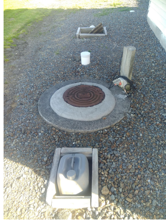
Existing Septic Tank
